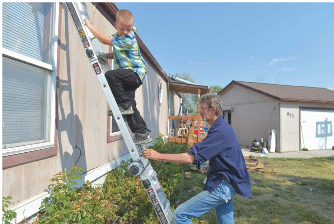
Justin Ryan follows his grandson, David, up a ladder as they replace shingles on their roof Thursday, Aug. 3, 2017.
